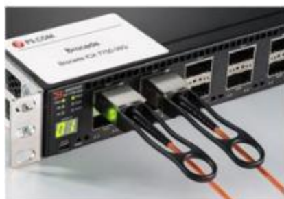
Brocade ICX 7750-26Q
